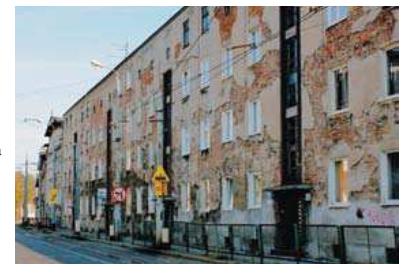
Fig. 4.17 Peeling facade of a tenement house in Władysława IV Street (Nowy Port, above) and fragment of wall riddled with wartime bullets in Sochaczewska Street (Wrzeszcz Dolny, below) Authors: Maja Grabkowska and Tomasz Strug
